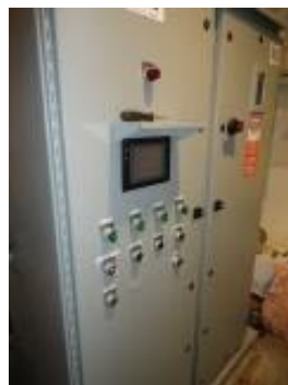
Pumpstation control panel
