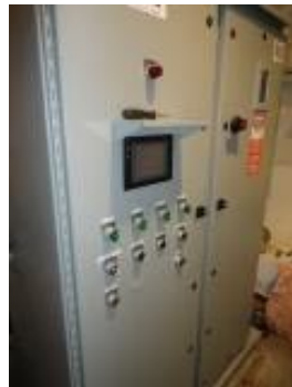
Pump station control panel
