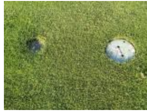
Irrigation sprinkler & wire box
