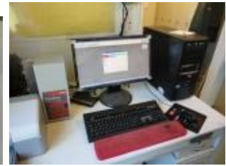
Irrigation central controller
